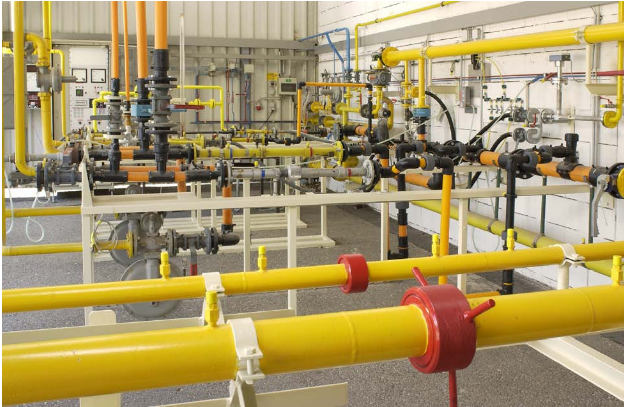
Figure 5: Natural gas test bench
