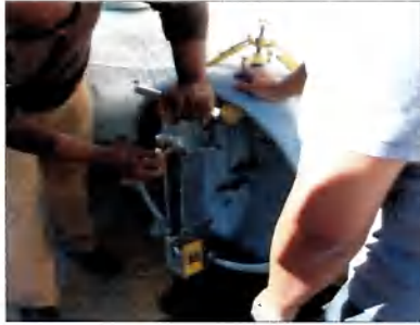
Chlorine B-Kit Installation
