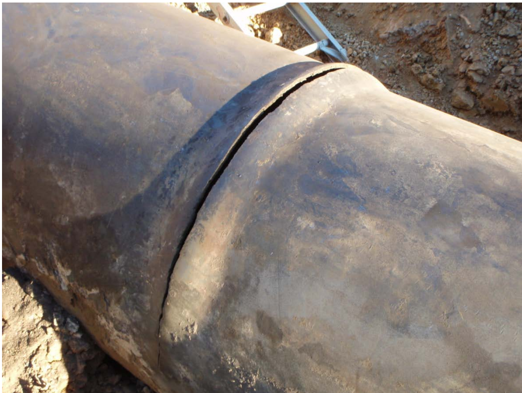
Figure C2 - Failed Wrinkle Bend
