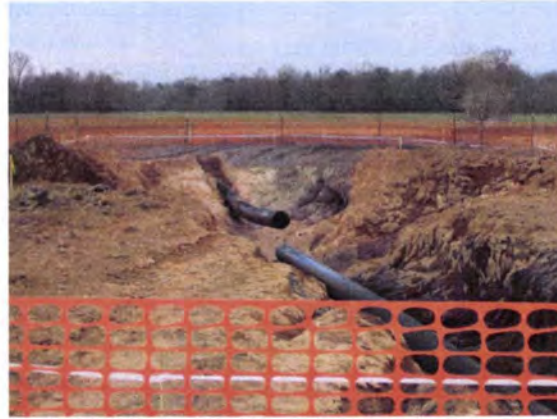
Failed 16-in South Main Line looking downstream
