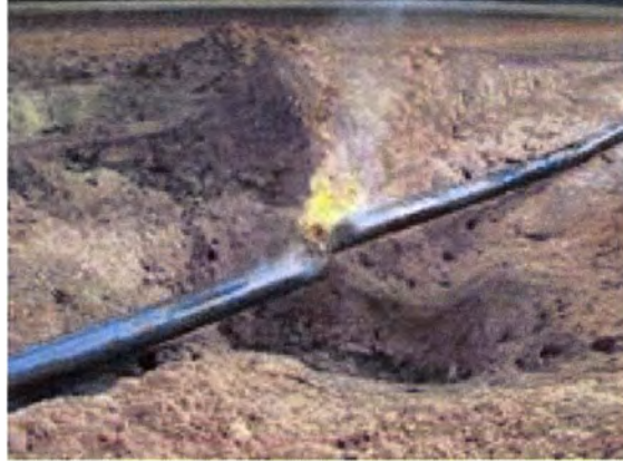
16-in South Main Pipeline after shut-in. Cover completely displaced by high natural gas pressure
