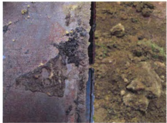
Weldcap intact on failed pipe.
