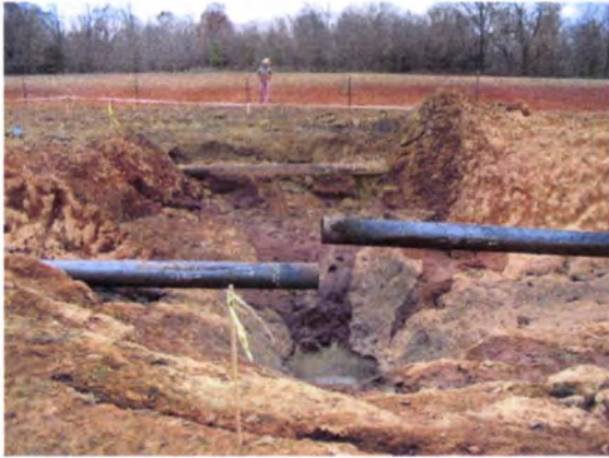
Failed 16-in South Main Line. Abandoned 12-in Montgomery to Columbus pipeline in background (partially exposed)
