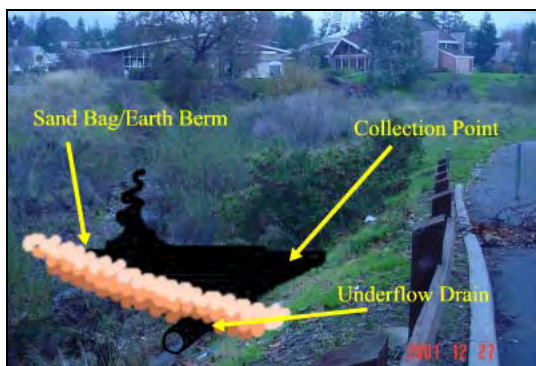
Figure C.8c Sandbag Underflow Dam
