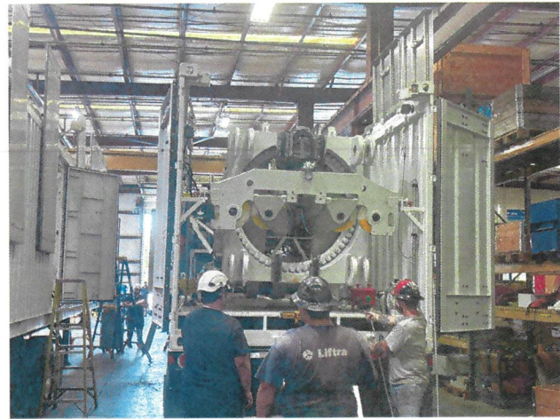
Figure 2. Rear opening of the enclosure with the LT1200 crane stowed inside.
