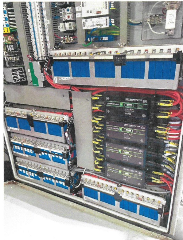
Figure 4. Integrated battery modules, BMS monitoring units, cabling, and LT1200 controls inside the Nacelle System.
