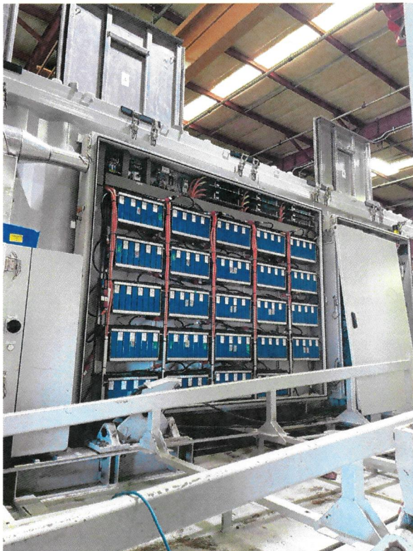
Figure 3. Fixed battery installation and dedicated structural/electrical modifications inside the LT1200 enclosure.
