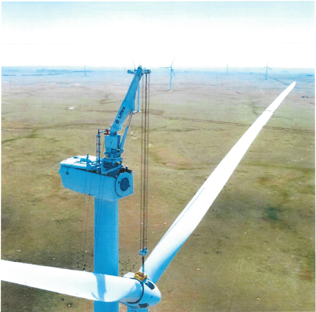
Exhibit Figure A-6. LT1200 LSHC deployed on a wind turbine, illustrating the operating purpose of the LT1200 system.
