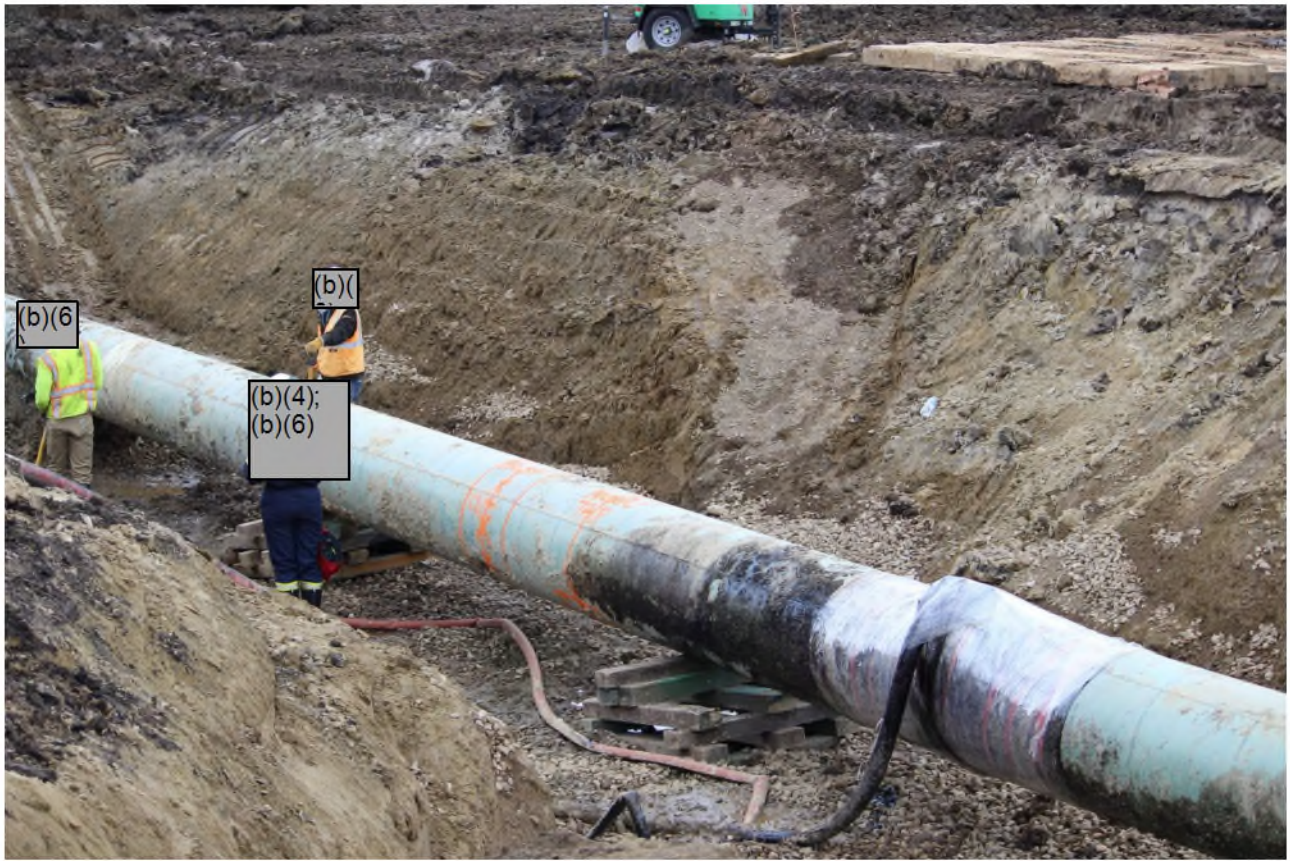
Figure 16. Fully excavated failure during the drain down operation. PHMSA AID Photo.
