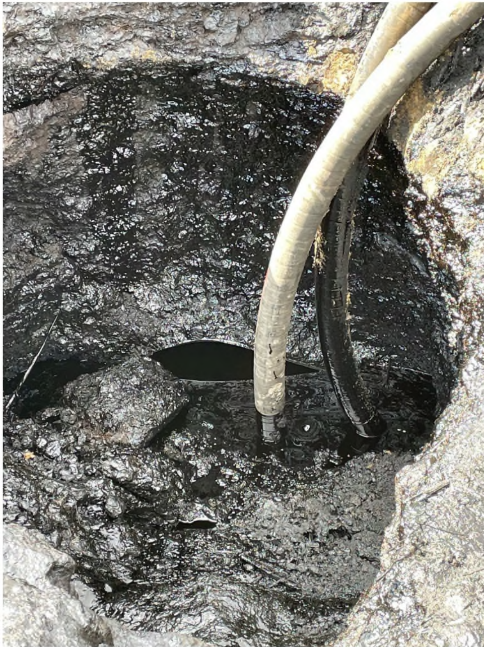
Figure 15. In Situ view of failure. PHMSA AID Photo.
