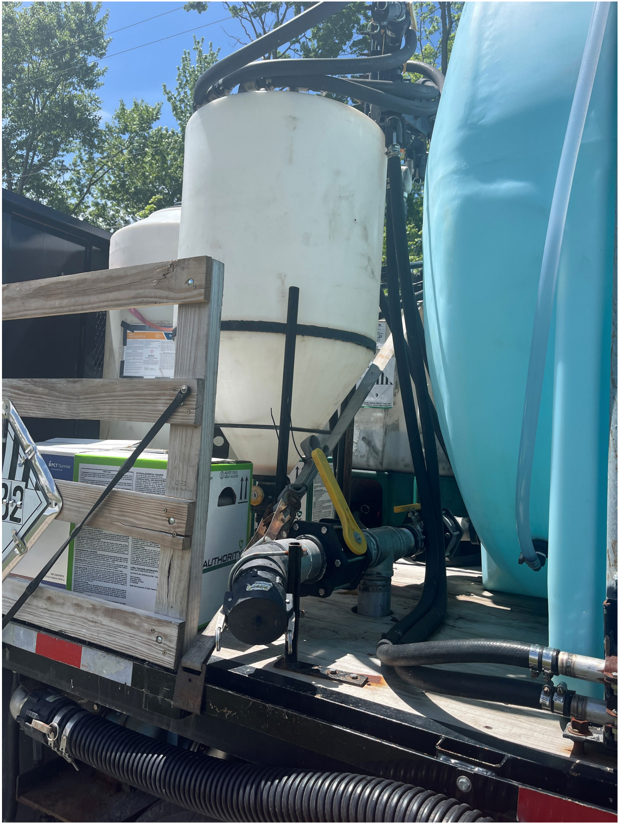
Close up of "inductor tank" and discharge pipe
