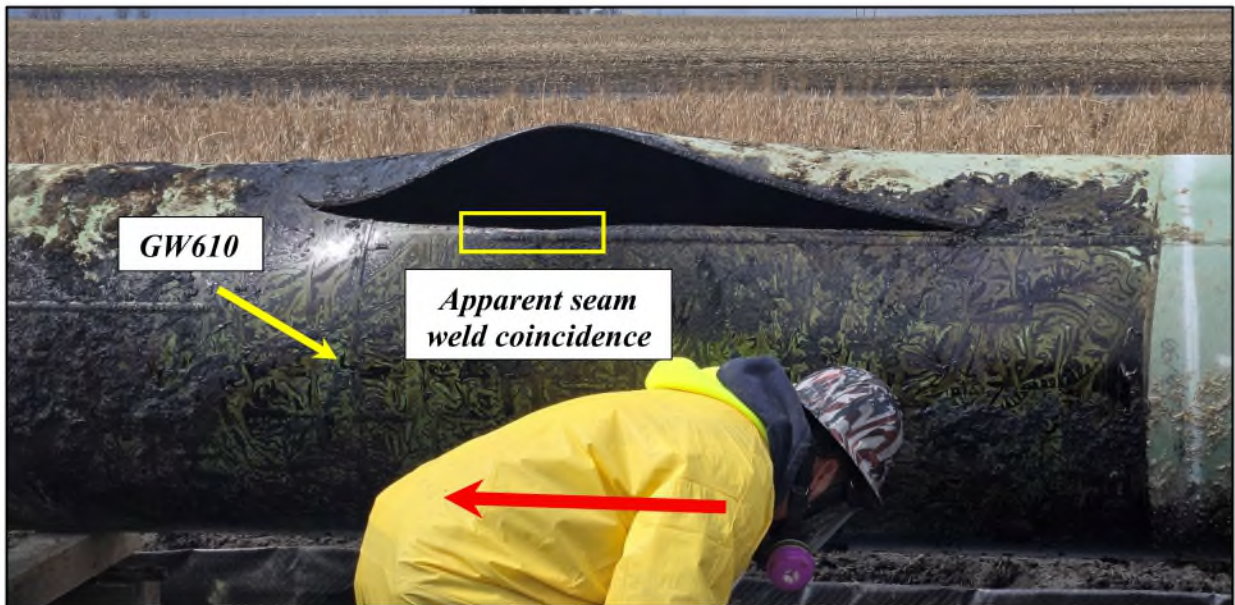
Figure 2 – Photograph of the rupture following removal of the plastic wrap covering. It was confirmed at this time that the rupture had a partial coincidence with the seam weld on the joint upstream of GW610, traversed GW610 and propagated in a clockwise direction in the base metal of the downstream joint. The red arrow indicates flow direction.
