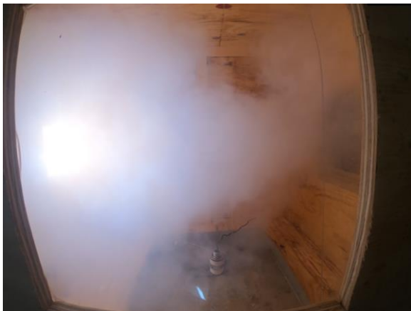
Picture 5: Stat-X 30E smoke box after activation
