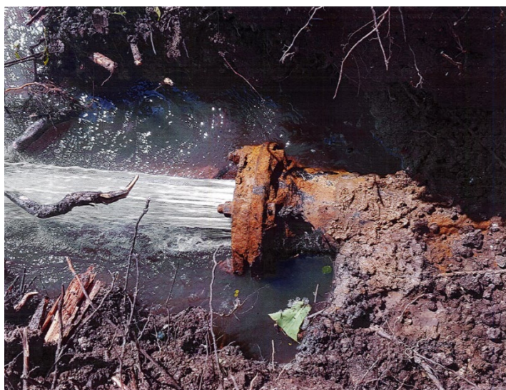
Figure 2-23: St. Parish water line being exposed from impacts from Hurricane Barry (Source: HMPU Committee)
