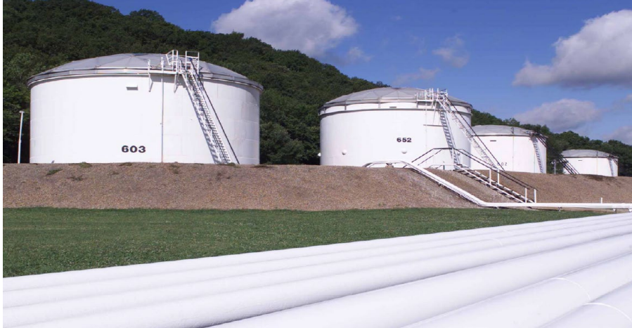
Figure 2 – API 650 tanks as part of a tank farm (Photo courtesy of an operator)
