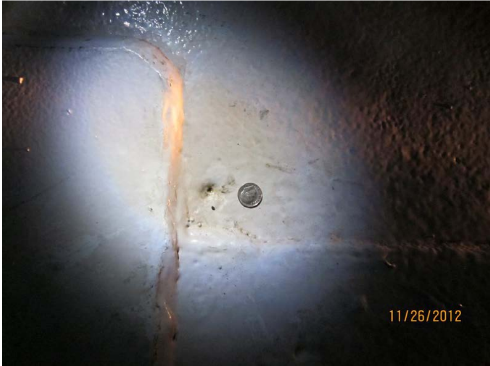
Visual indication of the through-bottom hole, 11/26/2012 (Magellan provided the photograph)
