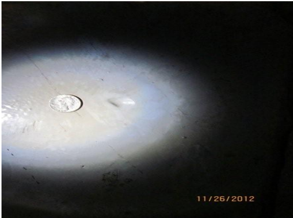
Visual indication of defect in close proximity to the hole, 11/26/2012 (Magellan provided the photograph)
