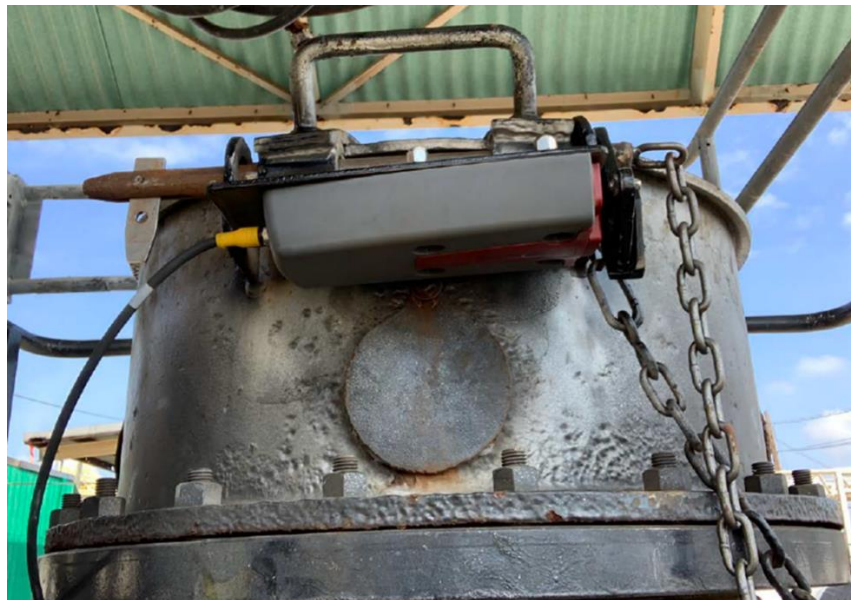
Figure 4.7 - Fully Installed Device
